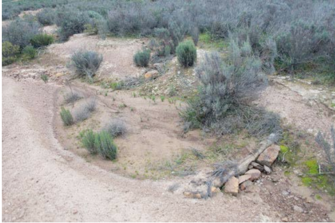
Rehabilitation of degraded land via a check dam at Avontuur in Namaqua District, Northern Cape
