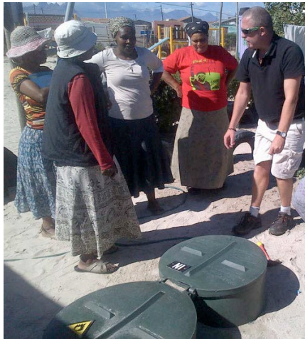
Project participants at Founders Educare Center in Cape Town installing a biogas digester and learning how it works
